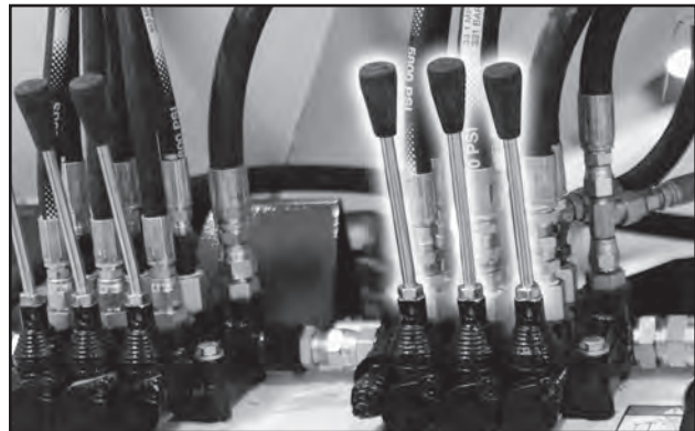
Fig 19 - Valves to Position Conveyor
